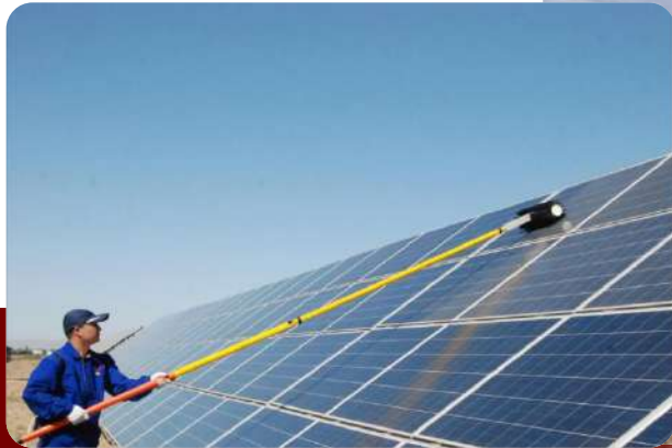
Cleaning the PV panels
